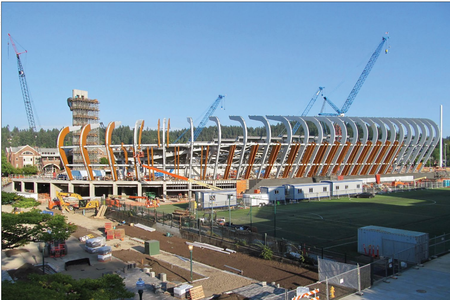
The new Hayward Field appears to be coming along quite nicely. Here's how things looked at the corner of Eugene's 15th & Agate on August 6.
